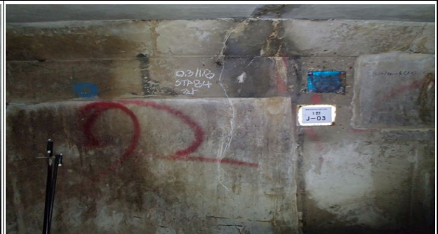
Type-1 J02~J03 균열
